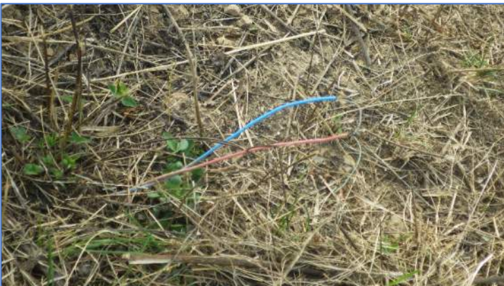
Photo 3, Point 3 Exposed wires at a point on the outer slope southwest of Phase 1.
