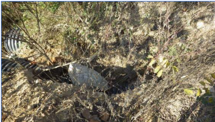
Photo 29, Point 29 Erosion at Phase 1 stormwater culvert ends upstream of West Sedimentation Pond along access road.
