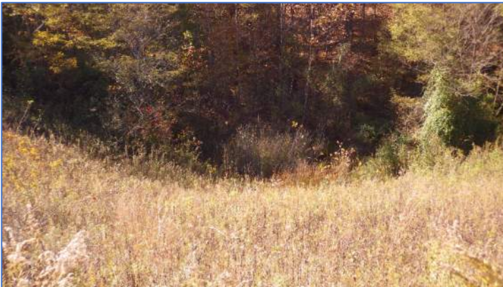
Photo 27, Point 27 Possible scarp on west side, exterior slope of the West Sedimentation Pond.
