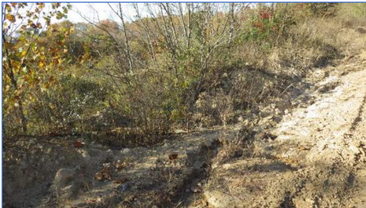
Photo 30, Point 29 Erosion gully at edge of road and close to Phase 1 stormwater culverts.
