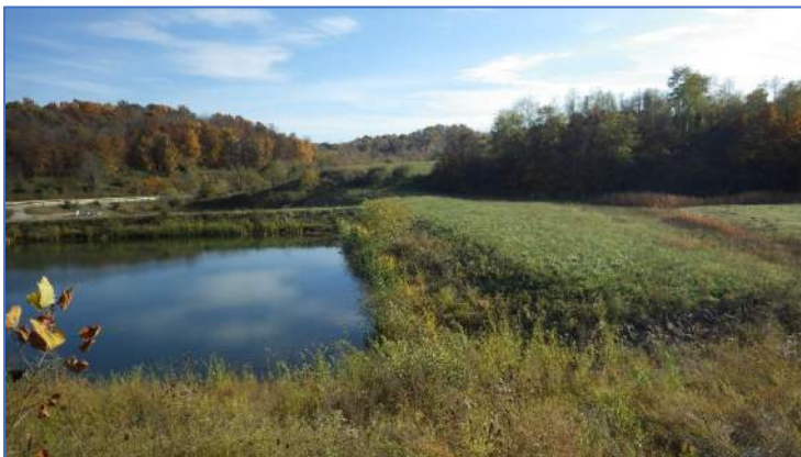
Photo 33 Erosion close to riprap spillway from Sediment Pond #1 (within Phase 4) into East Sedimentation Pond on left.
